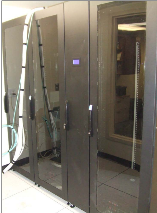
Front of cabinets and cooling unit
